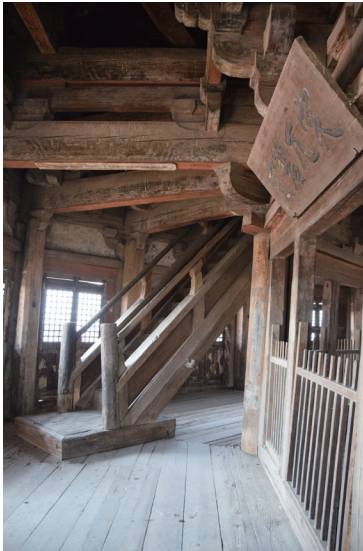
[Figure 44] Staircase leading to the fifth story of Yingxian Timber Pagoda. Liao dynasty, ca. 1056. [Photograph by Youn-mi Kim, 2016]
