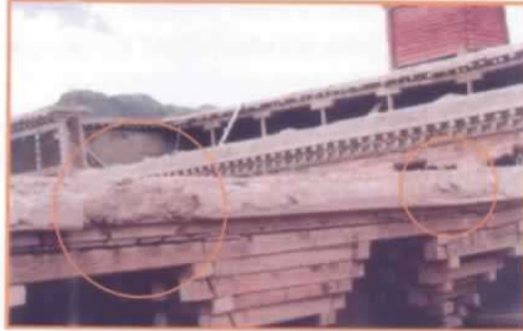
屋顶的横梁也出现裂缝。 The roof beams have also cracked.
