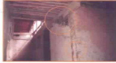
由于缺乏条件保养， 经过长期的风吹雨打， 墙壁破裂不堪。 Due to long years of poor maintenance, the wall has started crumbling.
