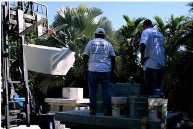
It's up and coming! Installers wait for it to get close enough to attach.
